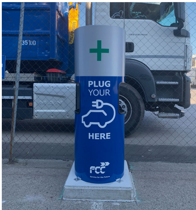
Charging station Himberg (Austria).
