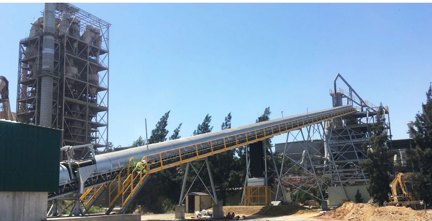
Biomass installation. Alcalá de Guadaíra factory, Seville (Spain).
