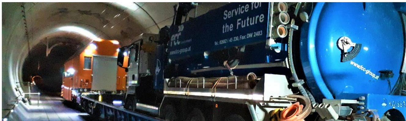
Drainage system cleaning tank.
