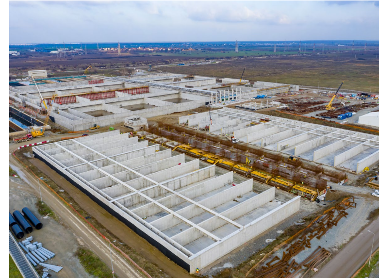
Wastewater treatment plant in Glina (Romania).
