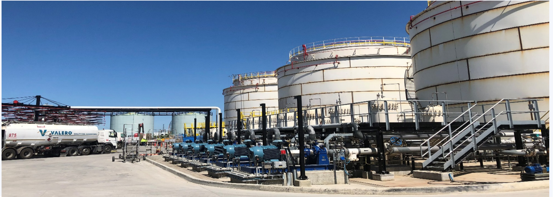
Industrial facilities Dublin Airport / Ireland Construction of three double-wall storage tanks of 5,000 cubic meters of capacity
