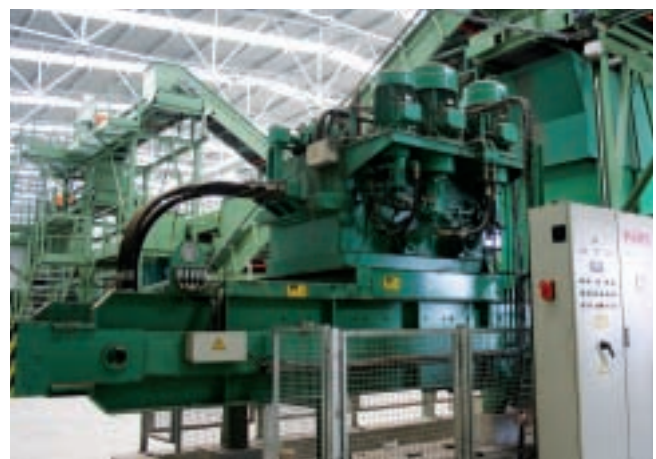
Solid urban waste treatment plant. Tudela. Navarra
