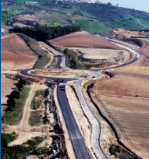
Medina Sidonia west relief road Section from dual carriageway A-38 to road A-390. Cádiz
