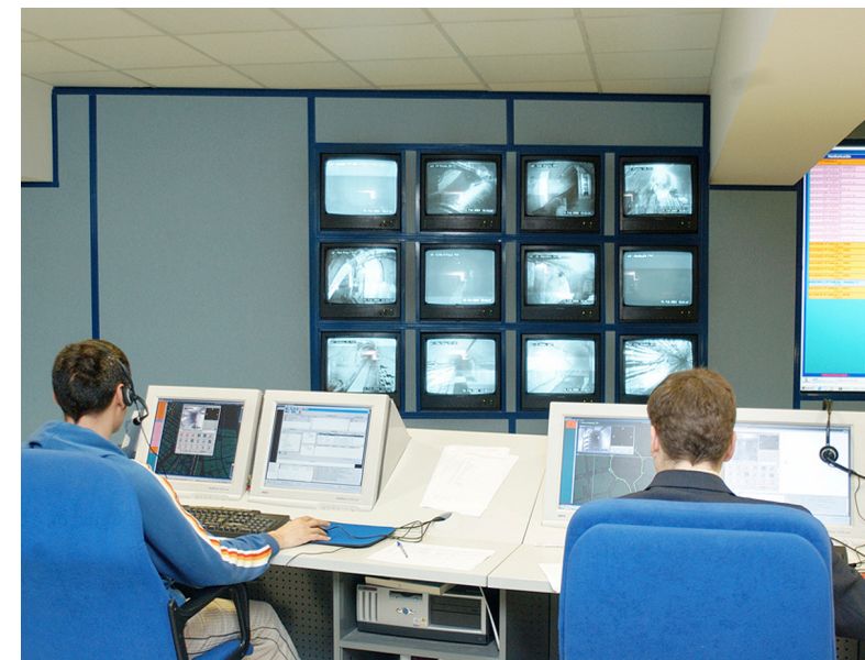
Control Center service tunnels, Madrid.
