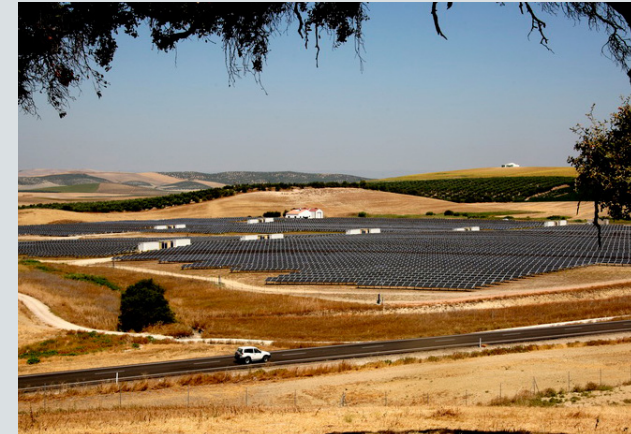
Photovoltaic farm in Córdoba
