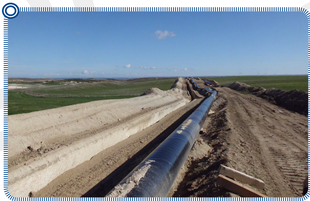
Yela-Villar de Arnedo oil pipeline.
