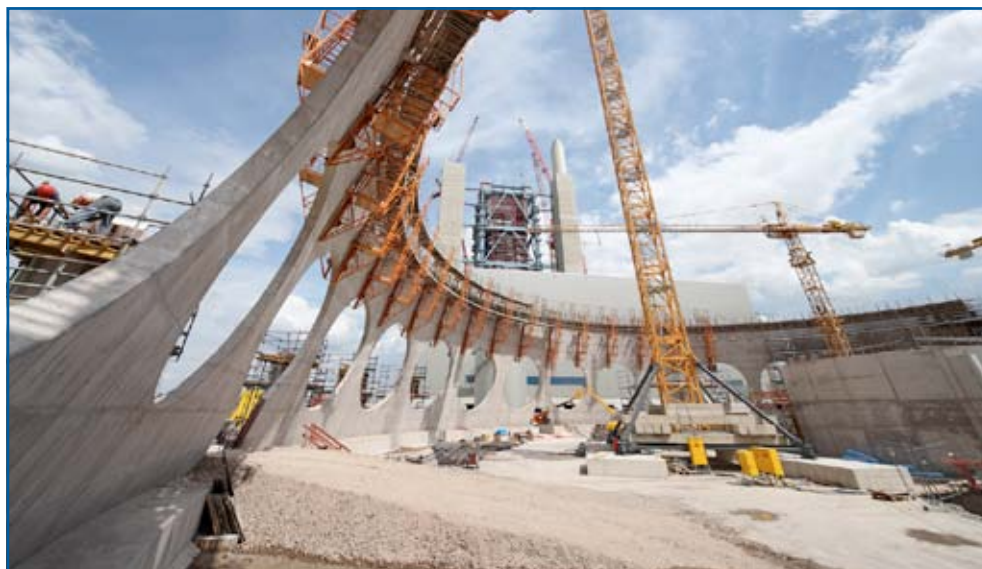
Karlsruhe Thermal Power Station (Germany)
