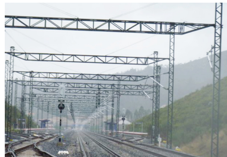
Catenary on the high-speed Atlantic Artery
