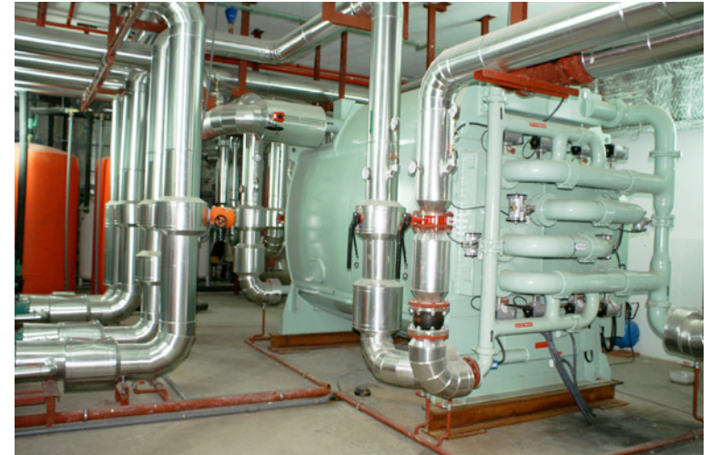
Absorption plant in an athletic complex, Madrid
