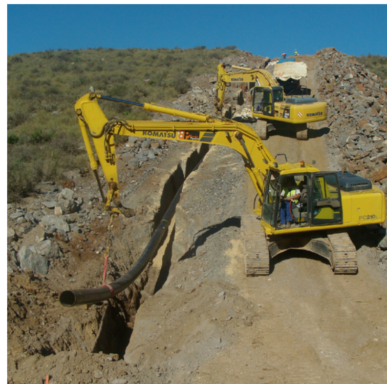
Alhama/Murcia oil pipeline
