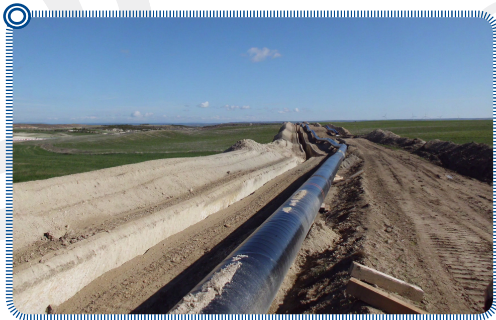
Yela-Villar de Arnedo oil pipeline.
