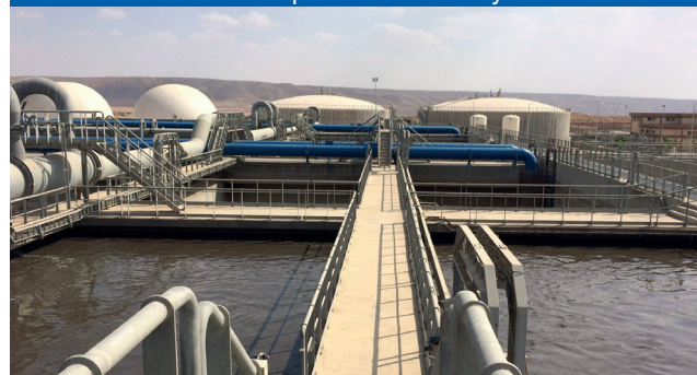
New Cairo Water Treatment Plant. Egypt.
